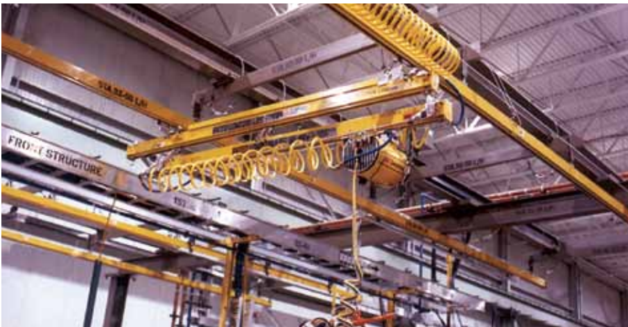
ETA-8 Body Shop Automation Crane and Runway System
